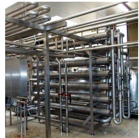
Example: New production line – food processing facility
